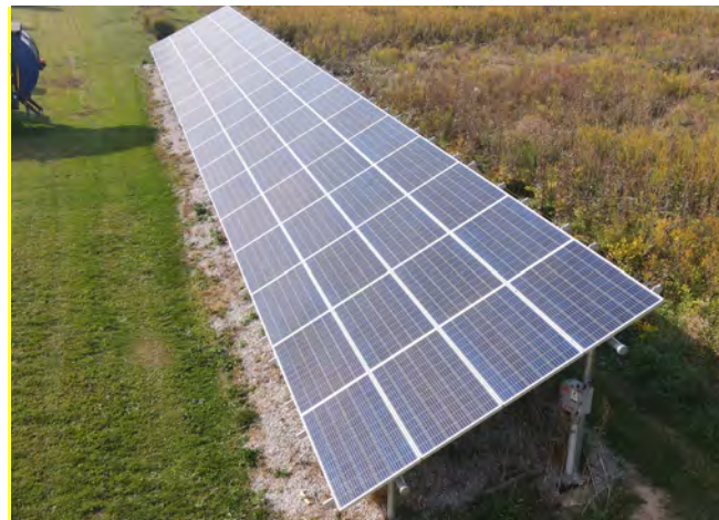
Solar panels power a recycling building on the Public Works campus, reducing the electric bill for the building by more than $5,000 a year.
