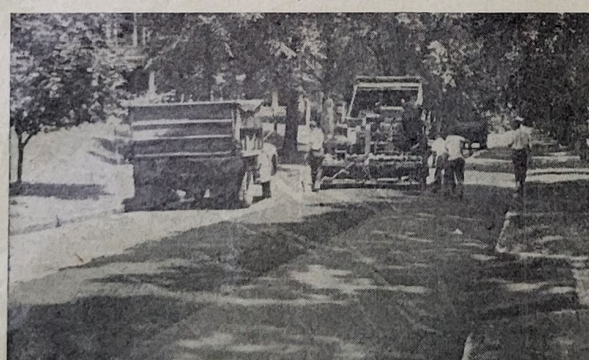
T-35 IN 1955 — A typical scene of the city's street division personnel resurfacing a city street with asphaltic concrete (T-35). Used on streets with adequate base and curb and gutter (such as old brick streets) this more permanent type of surfacing material results in lower annual maintenance costs. Other types of work include penetration
