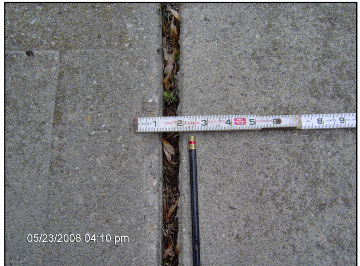
Open Joints Greater than 5/8"
