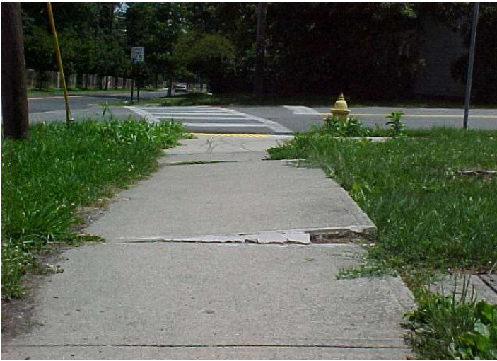
Tripping Hazards over 1/2"
