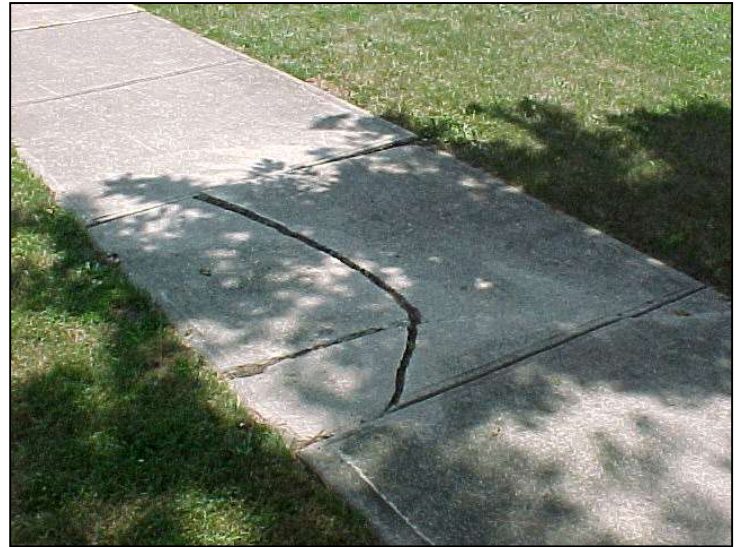
Cracked or Broken Sections
