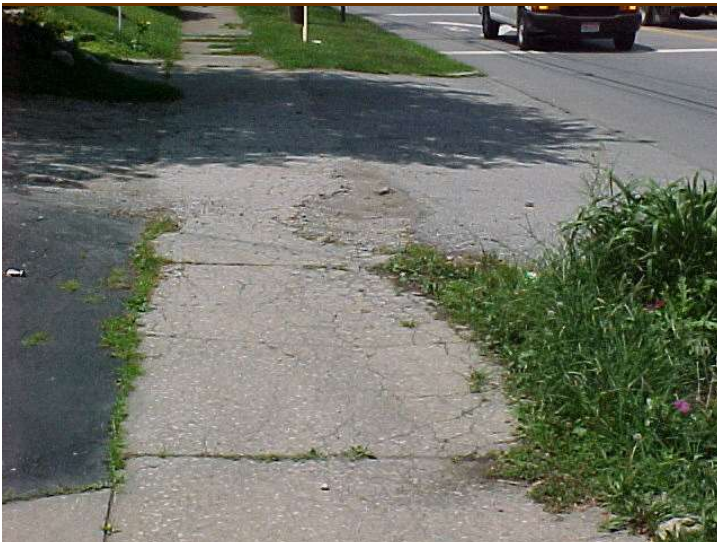
Deterioration of Sidewalk Surface
