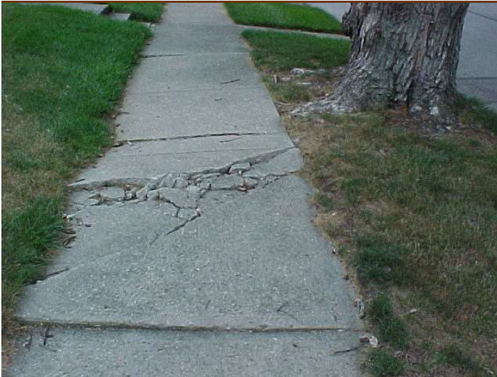
Tree Root Damage
