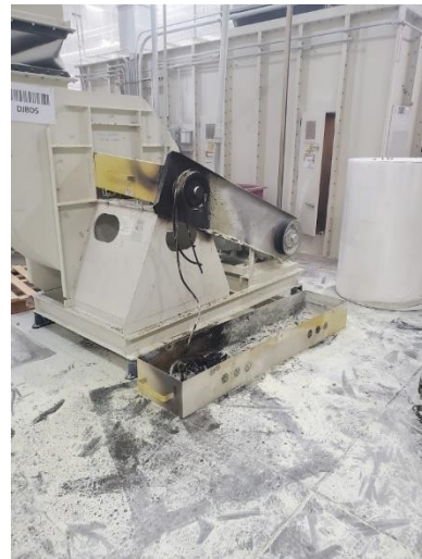
May 21 – Machine fire at US 42 Plant
