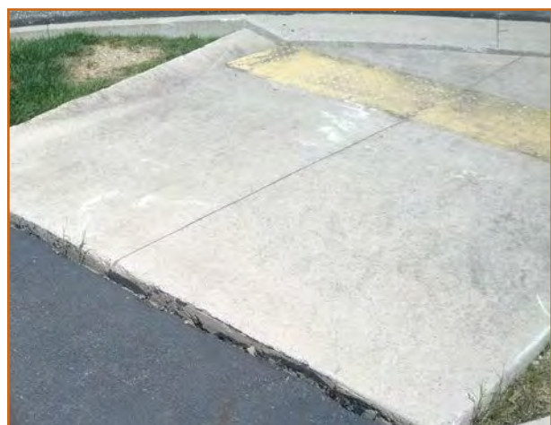
Figure 3-5: Here, the asphalt trail and curb ramp no longer meet.
