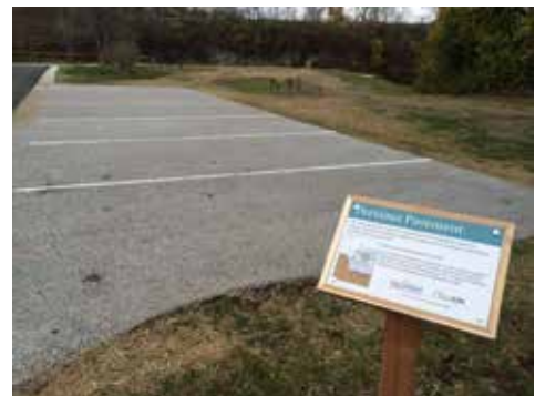
Permeable pavement has been installed at Blue Limestone Park helps to manage stormwater and provide numerous environmental benefits.
