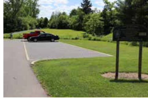
The City has used permeable pavers in parks, in ways that can be a model for private developers.
