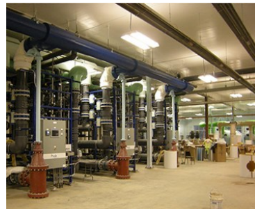
City of Delaware Water Treatment Plant
